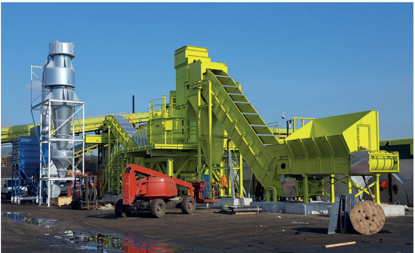
The recycling plant in the UK for processing automotive shredder residue (ASR) and electric and electronic scrap (WEEE) was still under construction here. It was planned and implemented by BHS-Sonthofen (©CMüller)
