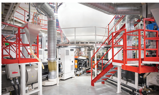
Rani Plast installation
