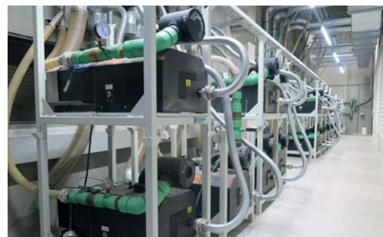
Picture 2: Glimpse of the machine room with the MINK claw vacuum pumps from Busch that supply various feed circuits with vacuum (Picture: Busch Vacuum Solutions)
