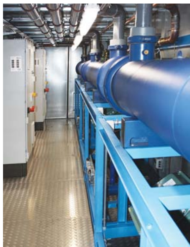
Three cooling units with a capacity of 400 kW each plus the respective control cabinets are installed inside the container – neatly and with a lot of space for service and maintenance works
