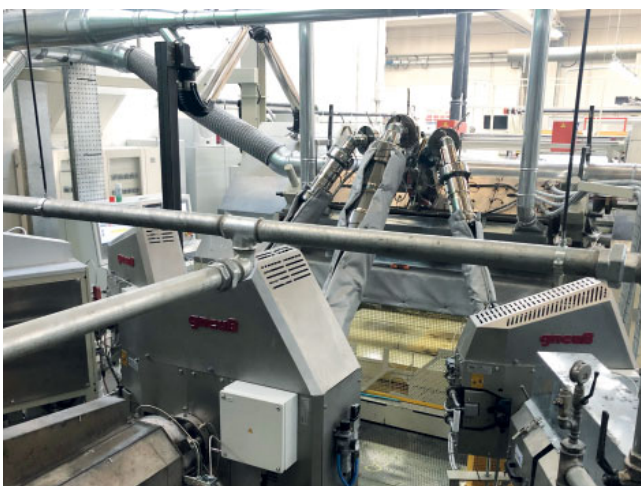
Sheet extrusion line at MP3 with three pressure- and process-constant Gneuss SFXmagnus melt filters
