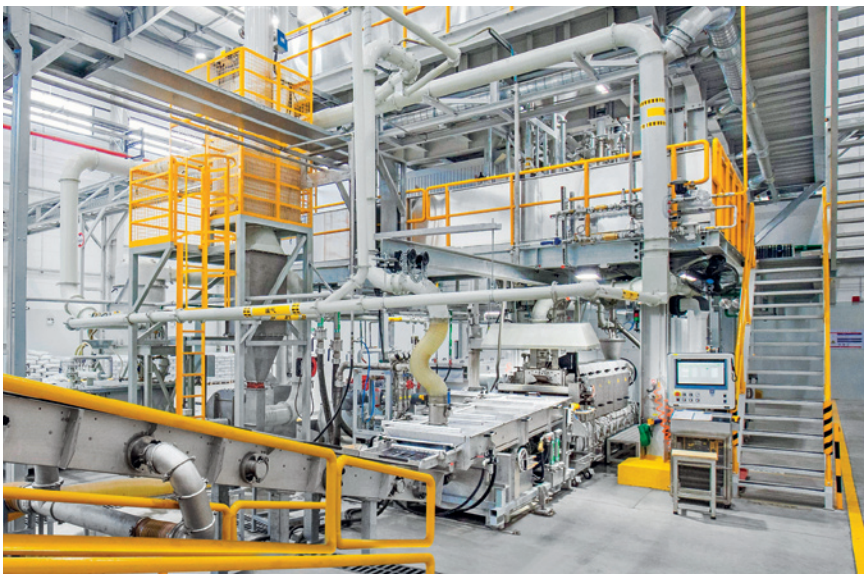
High-performance turnkey compounding line from KraussMaffei at Lanxess production site in Changzhou
