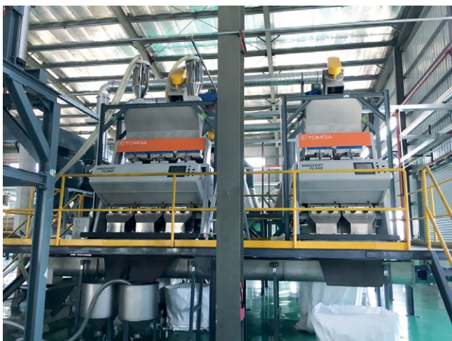
Flake sorters in recycling facility
