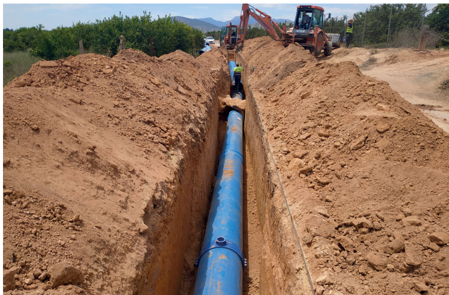
Installation of PVC-O pipes in the modernization project of the irrigation area of the irrigation community of the Tajo-Segura transfer of Librilla
