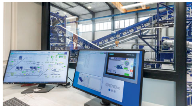
BHS Control Systems offers customized control systems for recycling plants
