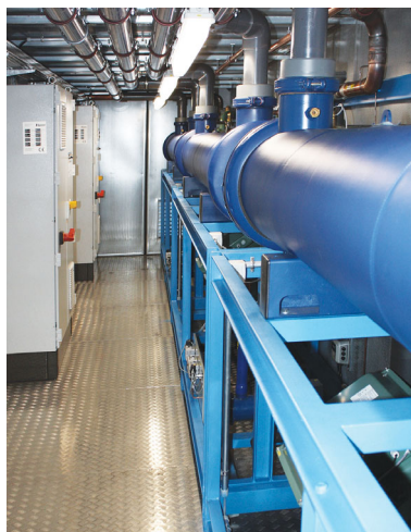
Three cooling units with a capacity of 400 kW each plus the respective control cabinets are installed inside the container – neatly and with a lot of space for service and maintenance works
