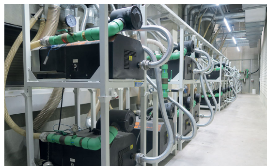
Picture 2: Glimpse of the machine room with the MINK claw vacuum pumps from Busch that supply various feed circuits with vacuum (Picture: Busch Vacuum Solutions)
