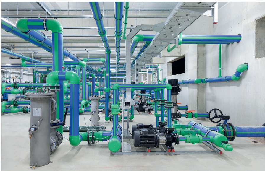
Picture 1: Pipelines from a cooling water treatment system in an industrial plant (Picture: aquatherm)
