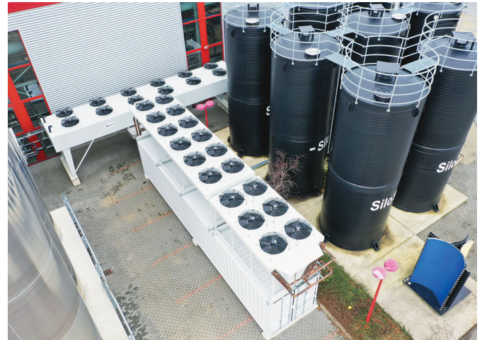
Cooling system container and dry coolers are placed between the new silos on the DRS outdoor area, where they are well protected
