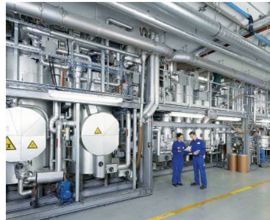
Bioplastic PLA pilot plant (Source: Sulzer)
