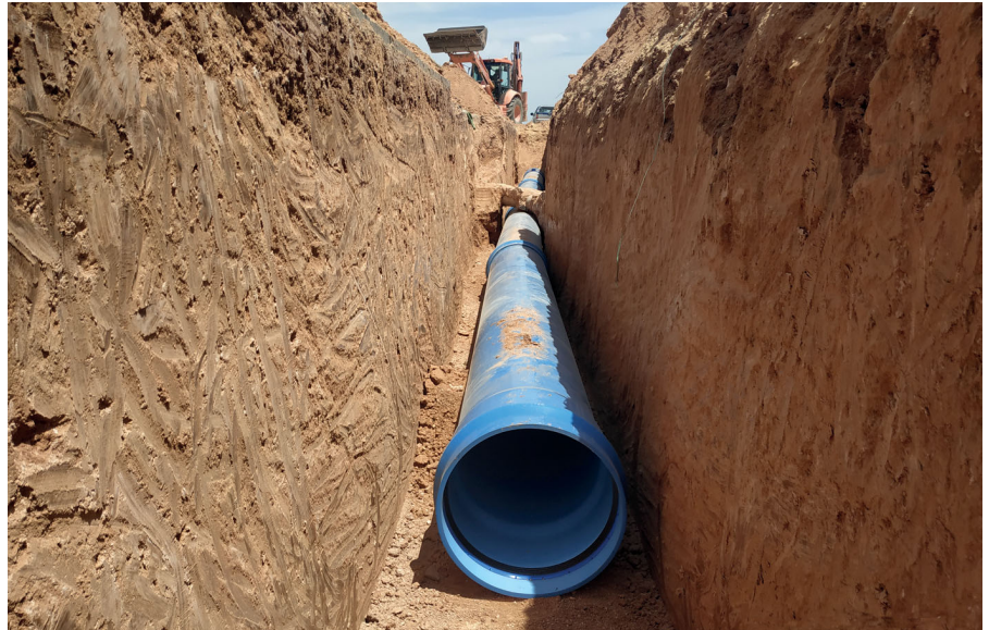
Installation of PVC-O pipes in the modernization project of the irrigable area of the irrigation community of the Tajo-Segura de Librilla transfer
