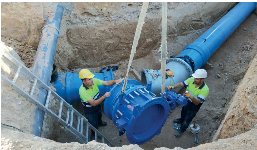
Installation of PVC-O pipes and special pieces in the modernization project of the irrigation area of the irrigation community of the Tajo-Segura transfer of Librilla
