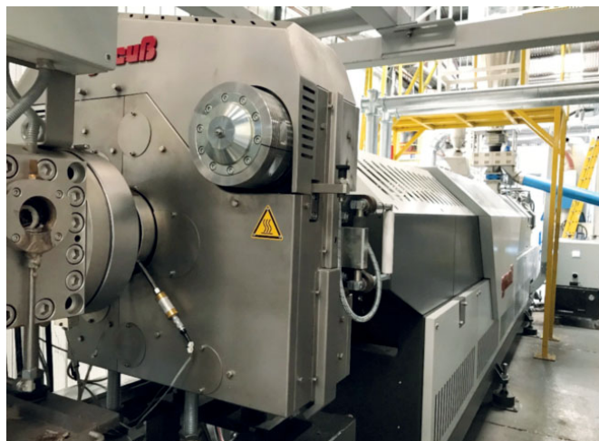
Retrofit solution in Southamerica
